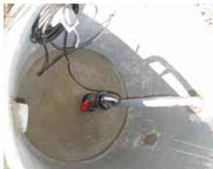
Station de relevage
